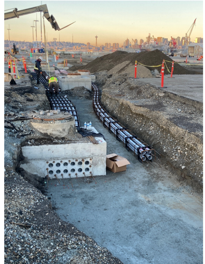
Secondary ductbank at substation
