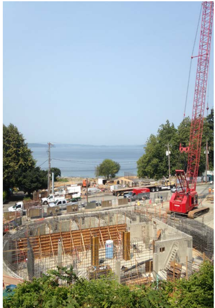
Fixing the crane boom over the weekend will help keep the project safe and on schedule.
